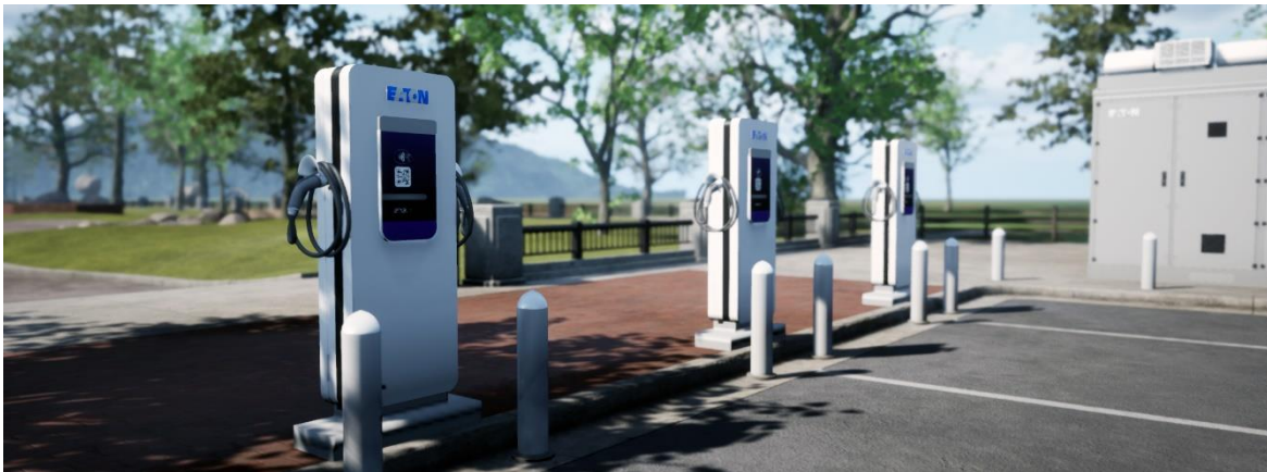
Figure 1. Eaton Charging Station with different EVSE. It can be noted how the EVSE also have many connectors as presented in the 1-3 tier model from the OCPP [9]. Extracted from https://www.eaton.com/us/en-us/company/news-insights/energy-transition/electric-charging/on-the-go-ev-charging.html
